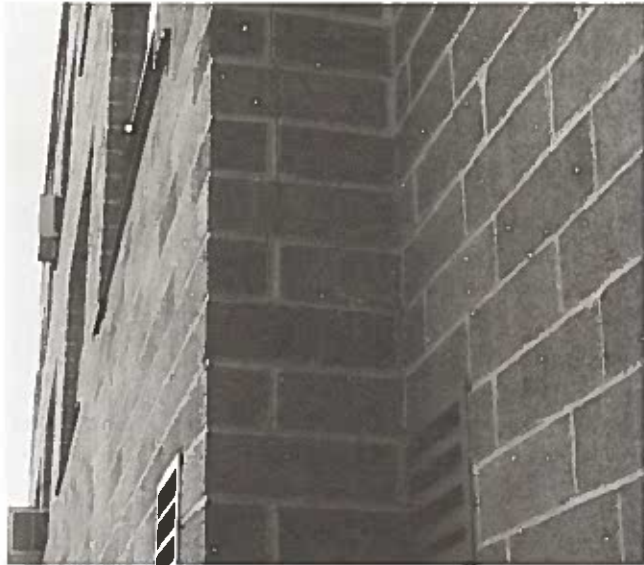
Crack at Offset
