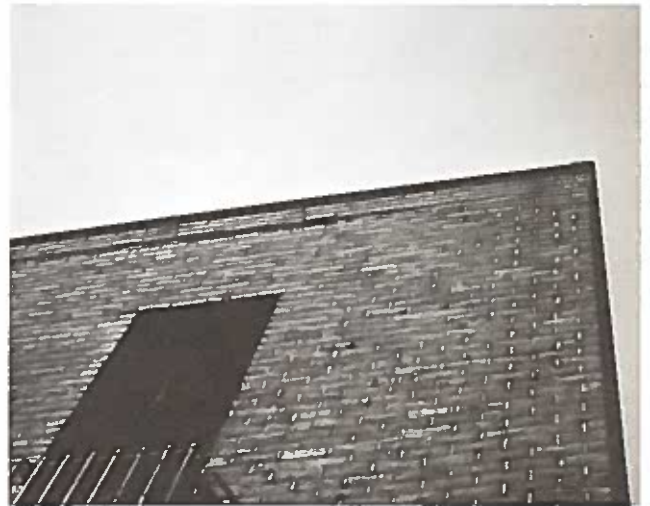
Bowing of Parapet Due to Expansion
