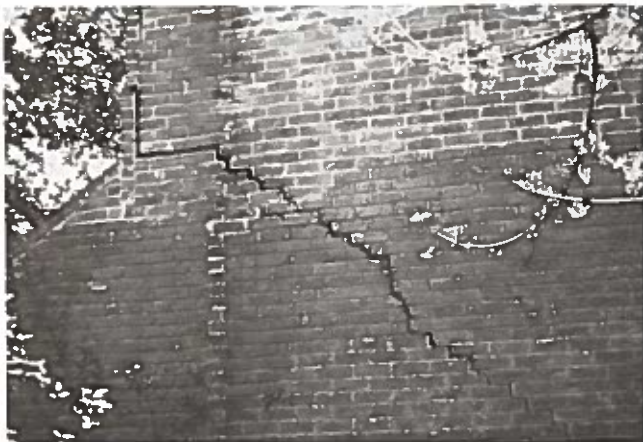
Crack Due to Differential Settlement FIG. 10
