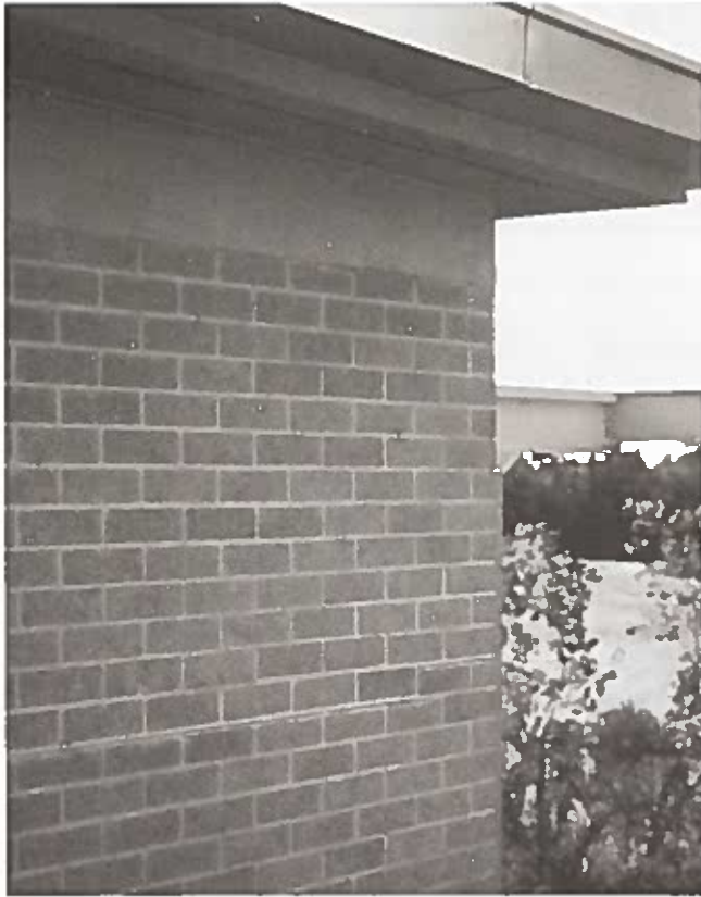
Crack Due to Curling of Concrete Slab
