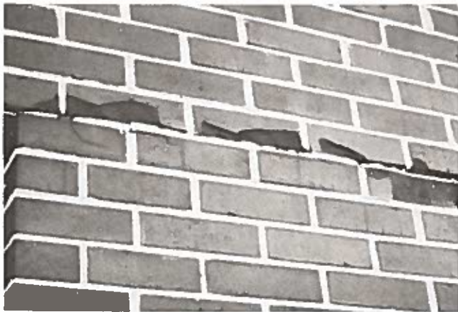
Spalling Due to Shortening of Structural Frame
