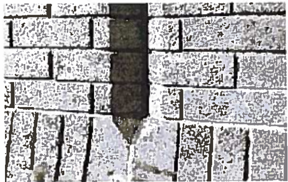
Photo 2 Accentuated Expansion Joint
