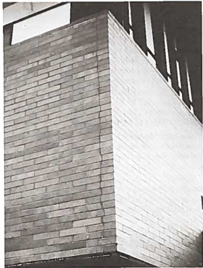
Crack at Corner
