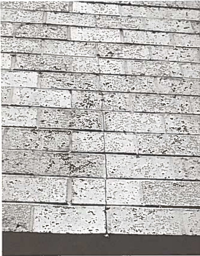
Crack Due to Deflection FIG. 9
